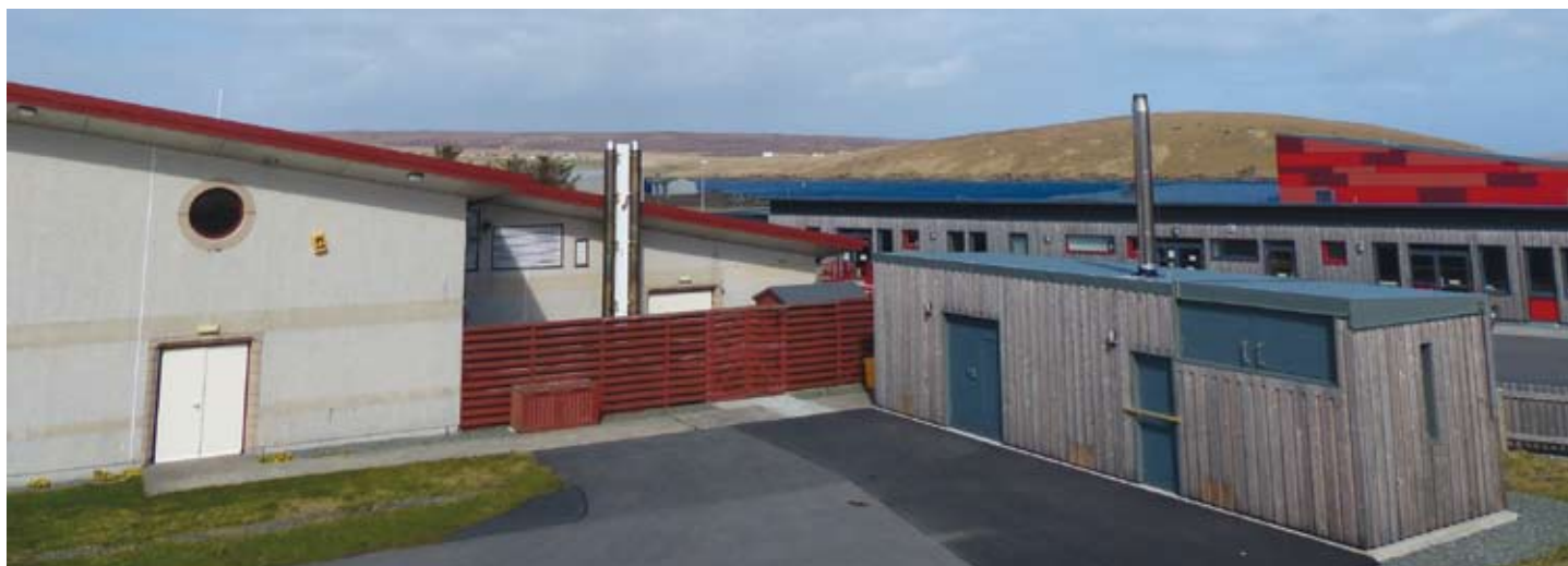
In the foreground is the biomass plant which was installed in summer 2012 to provide a more cost effective and environmentally friendly source of heating for the leisure centre and school.
